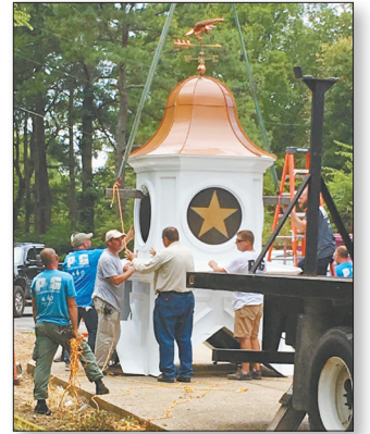
P&G Construction employees put some finishing touches on the cupola while on the ground (above) and in place on the roof (top). Staff photos TVM
