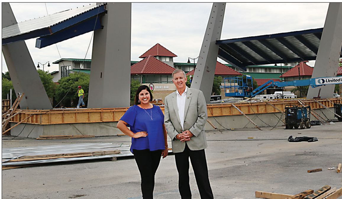
OVERSEEING PROGRESS: Present at the construction at the Tulsa State Fair are Amanda Blair, Tulsa State Fair manager and Expo Square COO, and Mark Andrus, president and CEO of Expo Square. In the background is construction for the greatly expanded Oklahoma Stage. Other improvements include the new Mega Barn, Pavilion exterior updates and improvements to the Tulsa State Fair entrance gates.
