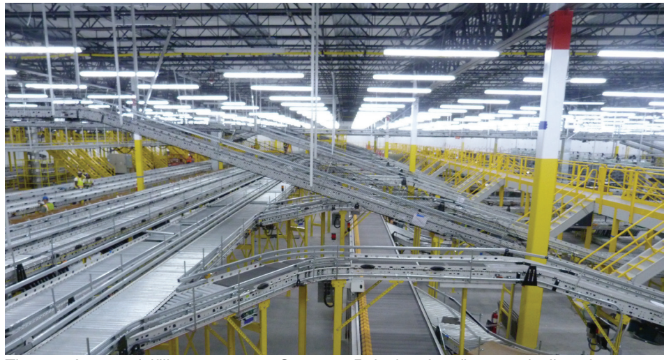
The new Amazon fulfillment center at Sparrows Point has four floors and miles of conveyor belts that can process up to 1 million items in 24 hours.
