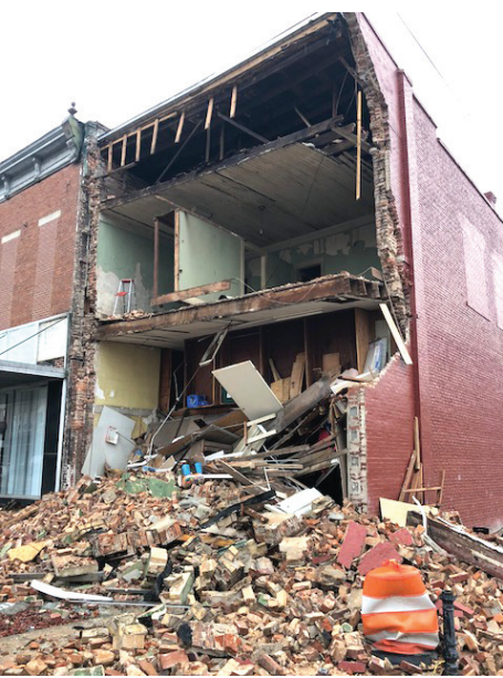
The front of this building at 127 North Jackson Avenue collapsed last Wednesday.
