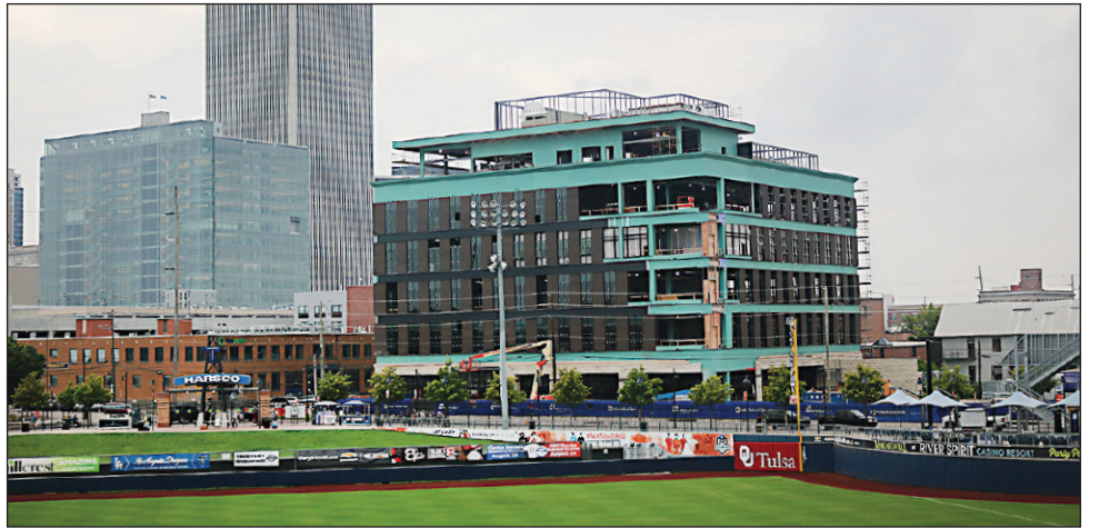
GOING UP: The new Vast Bank headquarters building across from ONEOK Field in downtown Tulsa is taking shape. Expected to open in December, the building will include a rooftop “In the Raw” sushi bar, rotating art installments and office space.
