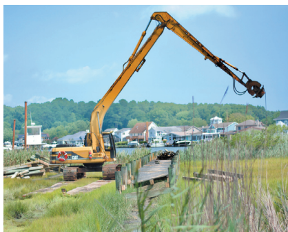
Fisher Marine Construction works to take down the remaining portion of the Whitetail Sanctuary crabbing pier.
