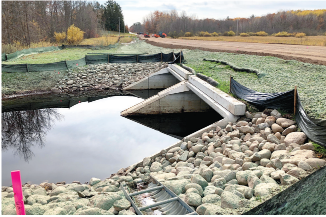
The Highway 47 box culvert bridge at Malmo Creek was replaced and the roadbed raised significantly. Due to rainy weather and delays, the road cannot be paved and is not yet open to traffic. Hopefully, it will open very soon.
