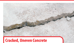
Cracked, Uneven Concrete
