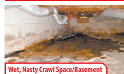
Wet, Nasty Crawl Space/Basement
