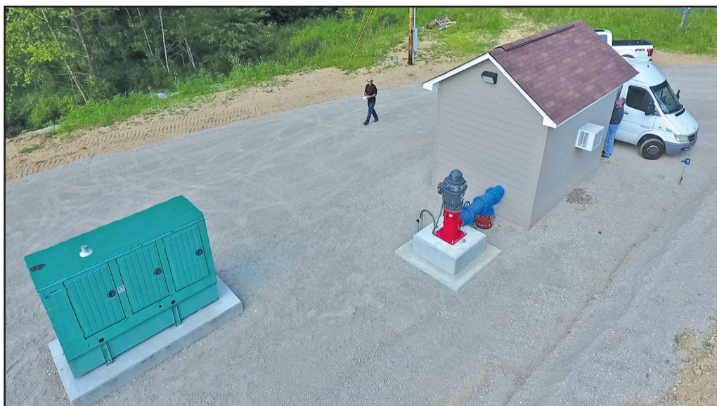
Water Well, Pump House and Emergency Generator
