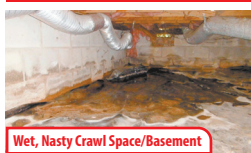
Wet, Nasty Crawl Space/Basement
