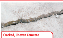
Cracked, Uneven Concrete
