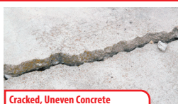
Cracked, Uneven Concrete
