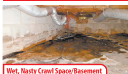
Wet, Nasty Crawl Space/Basement
