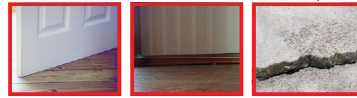
Doors Not Opening Properly
