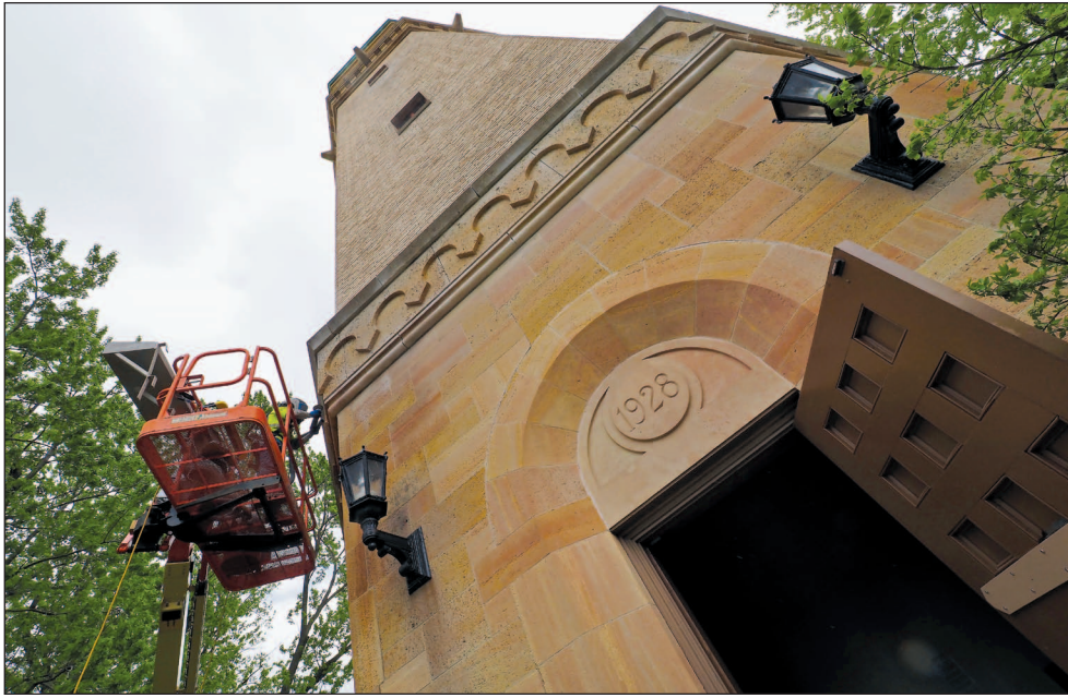
Things are looking up. Ryan Zappa of American Masonry Restoration grinds mortar joints on the side of the historic Highland Water Tower. The 92-year-old landmark is undergoing a face-lift with the help of a $250,000 grant from the Minnesota Historical Society. Masonry work, tile repair, improved site drainage, and window and door repair will continue through the summer. PHOTO BY BRAD STAUFFER
