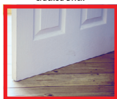
Doors Not Opening Properly
