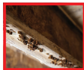
Mold in Crawl Space
