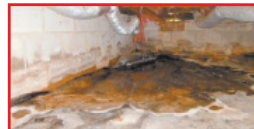
Wet, Nasty Crawl Space/Basement
