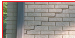
Cracked Brick or Drywall
