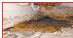
Wet, Nasty Crawl Space/Basement
