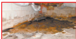
Wet, Nasty Crawl Space/Basement
