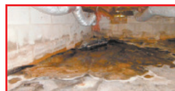
Wet, Nasty Crawl Space/Basement
