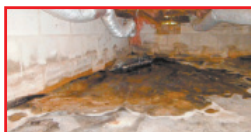
Wet, Nasty Crawl Space/Basement
