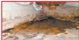
Wet, Nasty Crawl Space/Basement
