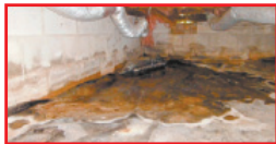
Wet, Nasty Crawl Space/Basement
