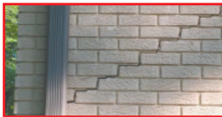
Cracked Brick or Drywall
