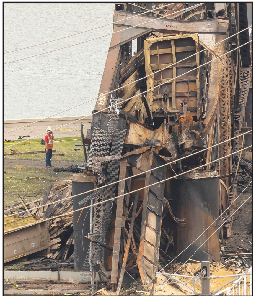
Top: Workers lower a replacement segment into place on the 108-year-old Salt River Union Pacific Bridge over Tempe Town Lake. Above: A derailment on July 29 destroyed the southernmost 150 feet of the span. That segment was blown up on Aug. 2 and quickly cleared so that reconstruction could begin immediately.
