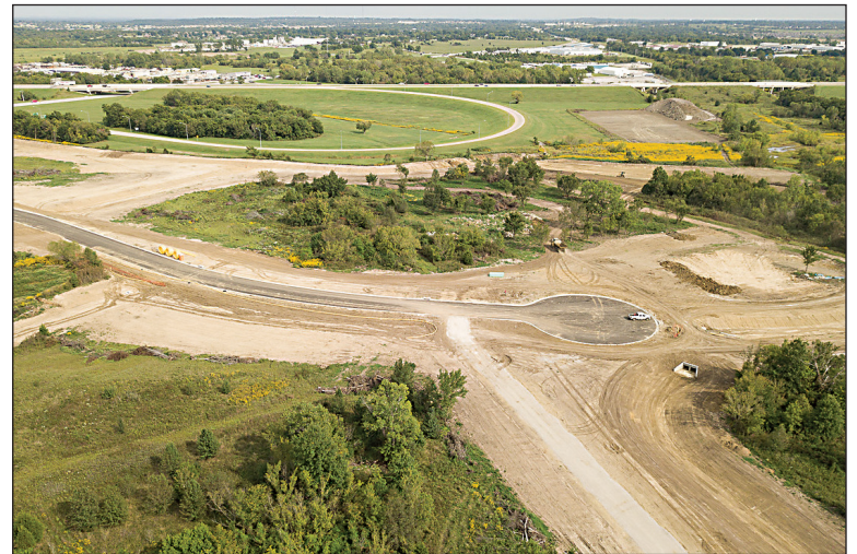
READY FOR ACTION: The Creek 51 industrial park is being called a business magnet that is expected to generate $1 million in ad valorem taxes per year when it is completed. It is located on the corner of the Creek Turnpike and Highway 51 and will include retail, office/warehouse, light manufacturing and distribution facilities.
