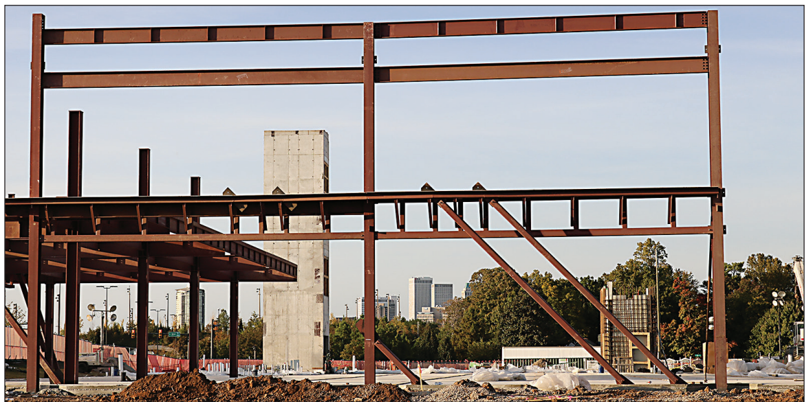
GOING UP: Construction of the Discovery Lab at Tulsa's Gathering Place is progressing for the scheduled opening in the fall of 2021. This photo was taken in early October as construction was beginning. The facility is located along Riverside Drive near East 31st Street at the south end of the Gathering Place.
