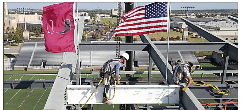
SIGNIFICANT PLACEMENT: The signed beam is placed at Tuttle Stadium. Additional improvements include a fine arts addition for the band program, new wrestling facilities and a new press box. The stadium is expected to open in 2021, followed by the fine arts addition in 2022.
