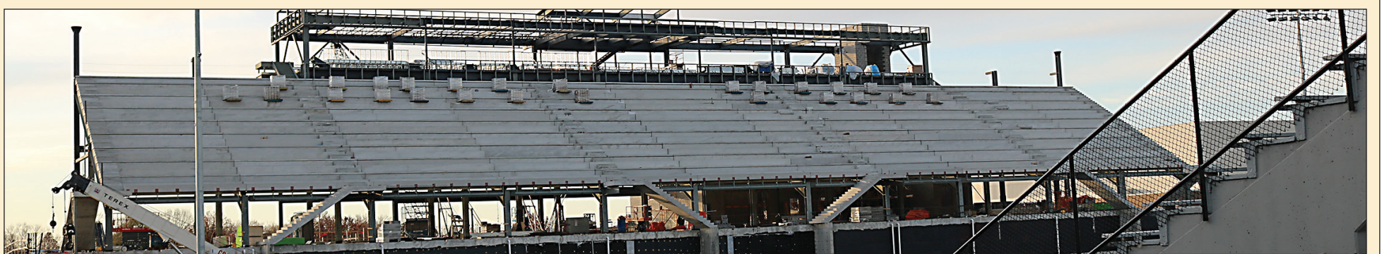
UNION STADIUM UPDATE: Construction of the west side of Union Tuttle Stadium, which began in the summer of 2019, is progressing. The stadium should be ready to re-open in the 2021 season. Updates will be published in the Union Boundary.
