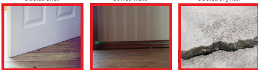
Doors Not Opening Properly
