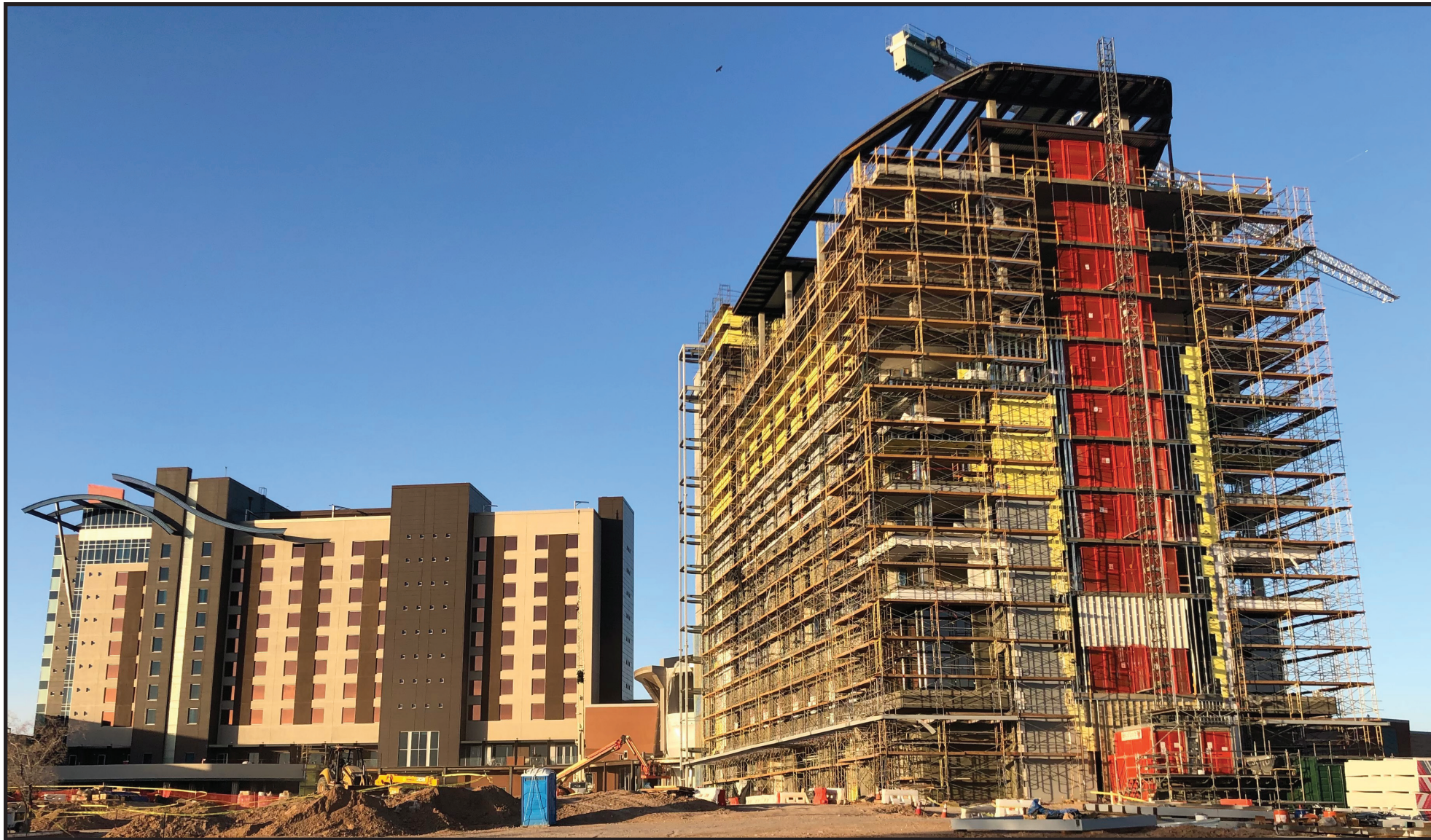
A second 11-story tower will nearly double room inventory at Wild Horse Pass Hotel & Casino.
