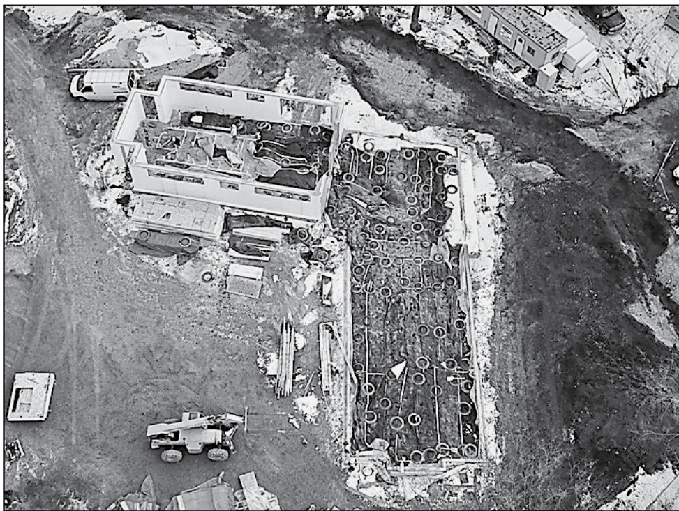
This aerial view shows progress on the Kohler Center for Marsh Education which is being constructed at the Sheboygan Broughton Marsh.
