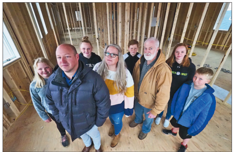
Lloyd's Pharmacy owner Jim Stage, his wife Cally, contractor Joe Beitler and Stage's children stand inside the drug store he is rebuilding at Snelling and Minnehaha avenues.
