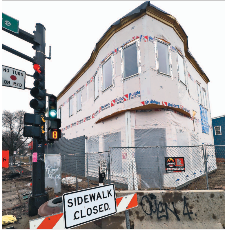
One of the most promising signs of rebuilding in Saint Paul is the new Lloyd's Pharmacy under construction on the southeast corner of Snelling and Minnehaha avenues—on the same site as the old Lloyd's, which was looted and burned to the ground on the night of May 28-29, 2020. PHOTO BY BRAD STAUFFER
