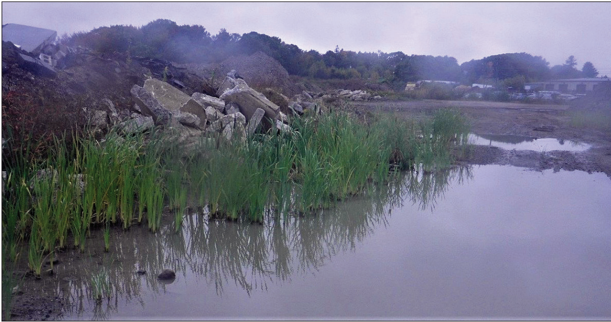
Mounds of fill material are seen in and near a wetlands area in Scarborough. Maietta Enterprises, Inc., Maietta Construction, Inc., and M7 Land Co. LLC will perform wetlands restoration and pay a fine under a consent decree with the U.S. Environmental Protection Agency and the US Department of Justice. (Photo courtesy of US EPA)
