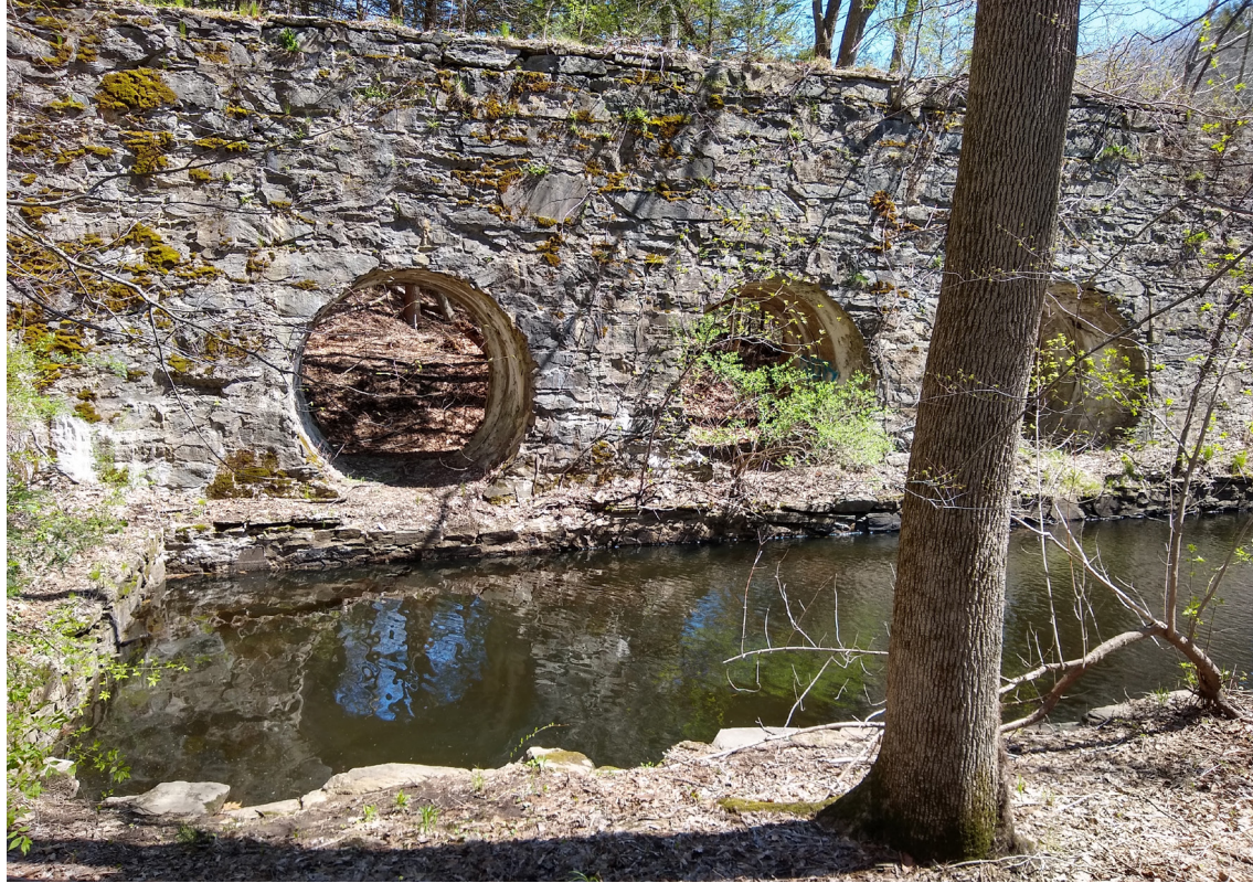
The unfinished Pomfret Power Company hydroelectric plant (1920) on the Quinebaug River in Pomfret. It was going to supply power for the Danielson Cotton Mills but may have been interrupted by the Great Depression. Photo by Donna Drasch.
