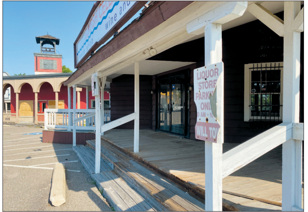
The former Sunfish Cellars is among the storefronts that have sat empty for three years now as redevelopment plans continue to languish at River Bluffs Center in Lilydale.
