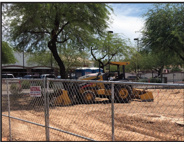
Bulldozers move large piles of dirt as construction gets underway on a Take 5 oil change shop at McClintock and Warner in South Tempe. — Wrangler News photo by Lee Shappell
