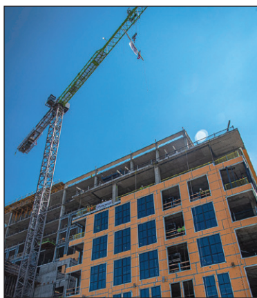
GOING UP: The final beam for the WPX building flies high during the topping out ceremony.
