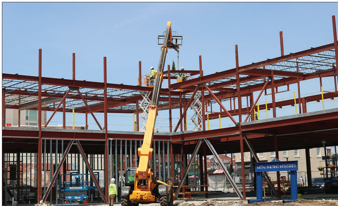
GOING UP: Members of the Manhattan Construction team top out the Brown-Kimbrough Arts Center for Creative Arts after the topping-out ceremony June 17.
