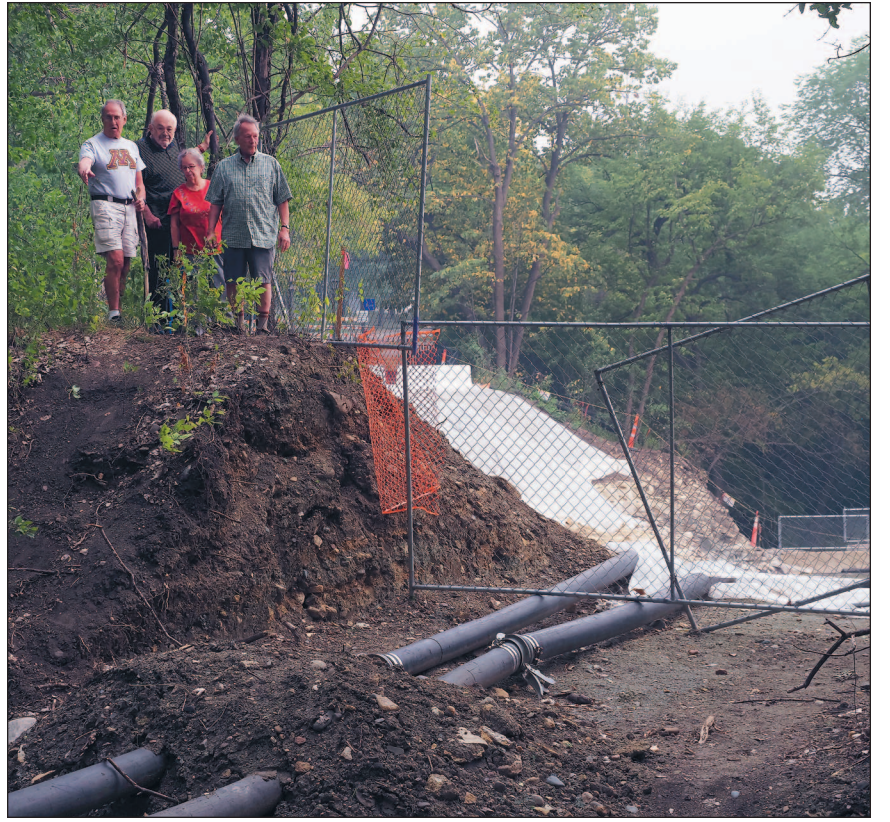
Highland Park residents Jim Ginther, Wy Spano, Marcia Avner and Jim Winterer survey the on-going work on the pedestrian tunnel underneath Mississippi River Boulevard that has closed that throughfare just south of the Highland Bridge development. PHOTO BY BRAD STAUFFER
