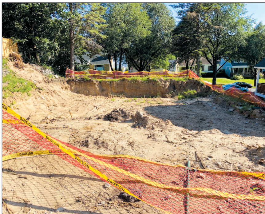
A view from the alley of the lot at 1945 Rome Ave. after the removal of the original rambler.
