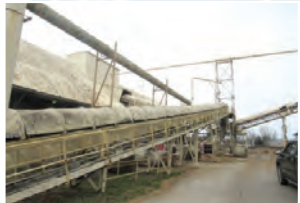
Large Amount of Concave Belt Conveyors
