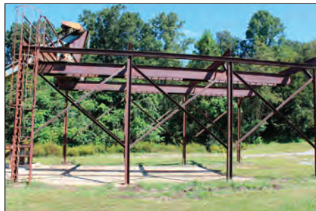
OVERHEAD TRUCK LOADING SYSTEM
