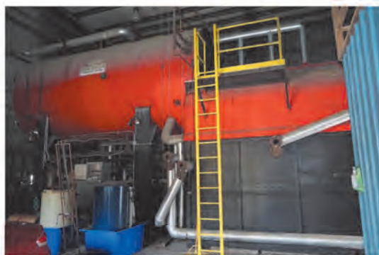
1992 Industrial Wood Boiler
