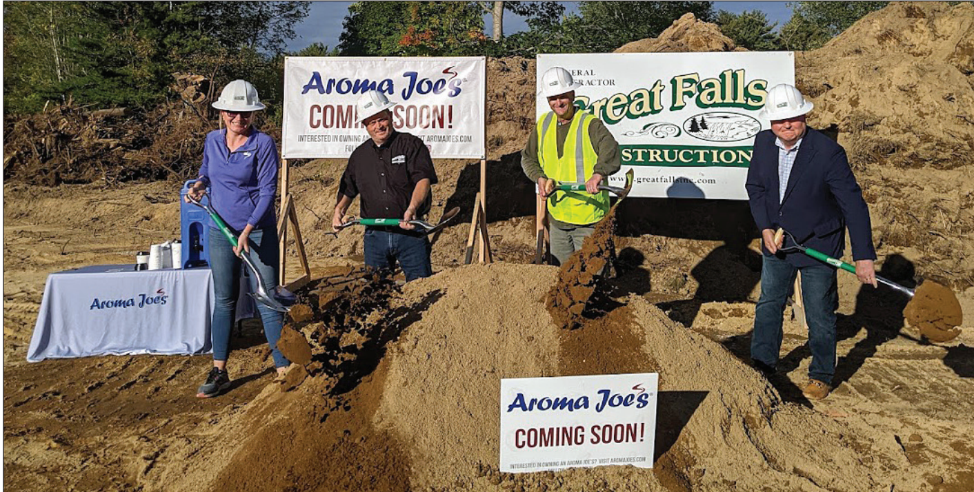
Great Falls Construction of Gorham broke ground last week on the site of the first Aroma Joes in Scarborough. Completion of the 1010 square foot facility is expected in early 2022. (Photo courtesy of Great Falls Const.)
