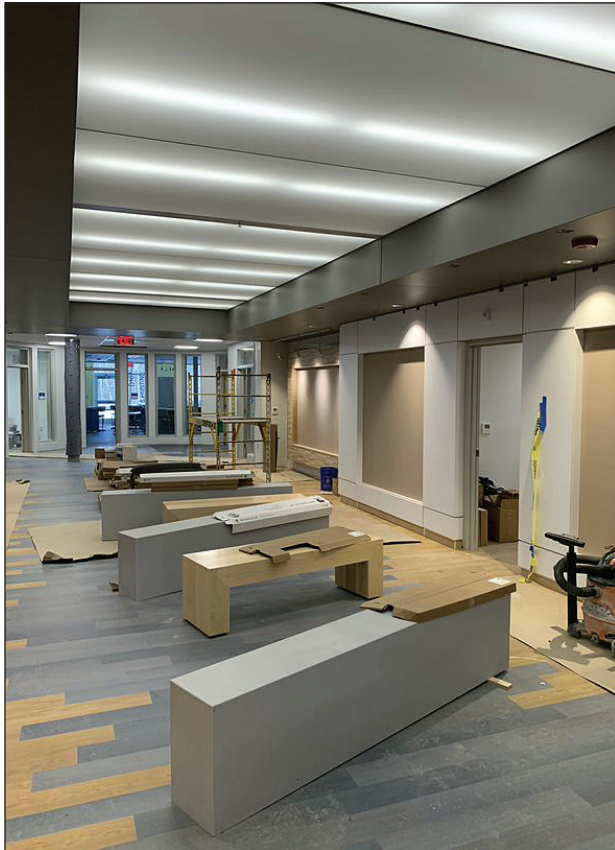
The first floor corridor is designed as a gallery space to showcase work created in the surrounding art rooms.
