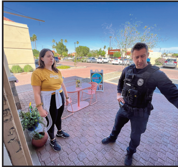
Karly Olson and Tempe Police Detective Ryan Cook inspect the front door of The Energy House, where three windows were broken as a burglar gained entry overnight and grabbed the cashbox.
