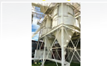
Several Dust Collectors
