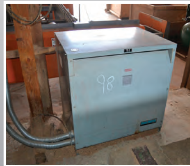
Acme 150 KVA Transformer
