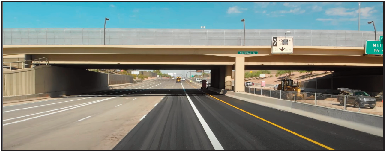
Eastbound lanes of U.S. 60 under McClintock Drive were the first to reopen after a water main ruptured May 7 and caused severe flooding that damaged the freeway surface. – Arizona Department of Transportation photo
