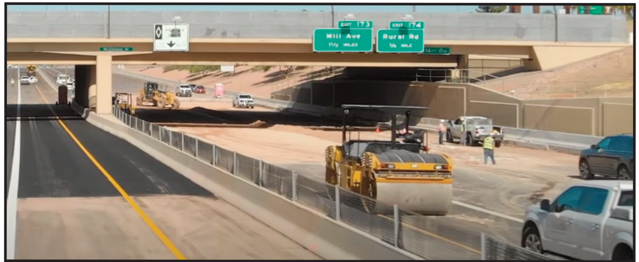
Work continues to rebuild westbound flood-damaged lanes of U.S. 60 under the McClintock Drive overpass after a break in a water main May 7. — Arizona Department of Transportation photo
