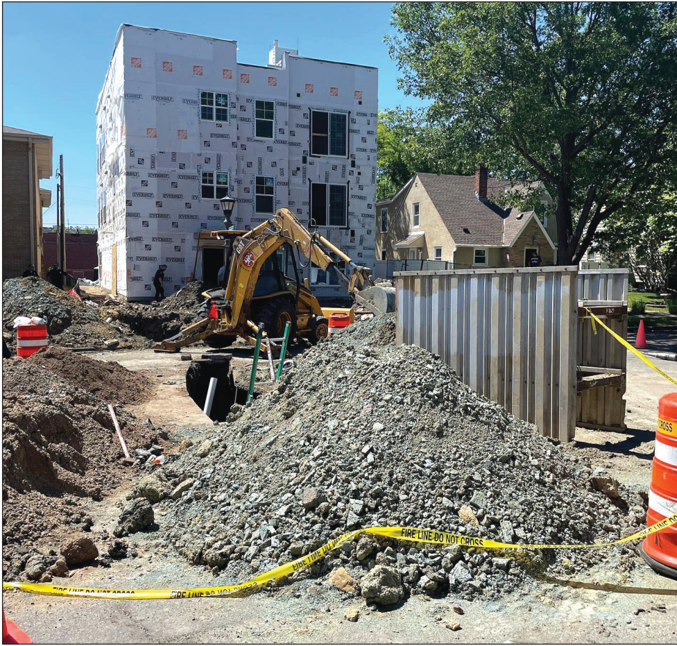
Firefighters worked through the night to recover the bodies of Bob Brandtjen and Jeff Jeanetta, who perished during a trench collapse on June 17 while working on a water and sewer project in front of an apartment building under construction on Mount Curve Boulevard. SAINT PAUL FIRE DEPARTMENT PHOTO
