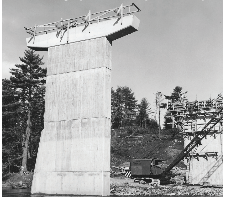
Before the Auburn and Lewiston Turnpike Exits opened in December of 1955, H.W. Hinman, Inc. of North Anson took charge of building the Androscoggin River Bridge.
