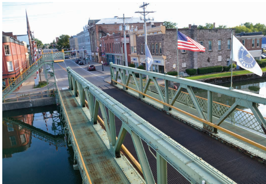
Photo by Tom Rivers: The Main Street lift bridge, shown on Wednesday evening, will be closed Oct. 17 for a major rehabilitation of the bridge that is scheduled to take 18 months.
