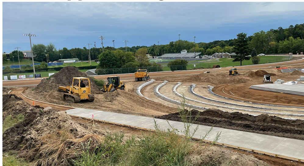
A view of the new Mississippi Landing Trailhead Park under construction with the Brainerd High School football stadium in the background and part of the amphitheater on the right.
