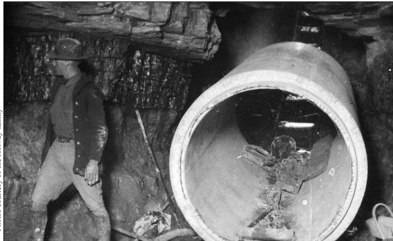
THE VERDIGRIS TUNNEL: The Verdigris tunnel required a subterranean excavation seven hundred feet long primarily through solid limestone creating a cave seven feet in diameter, large enough for the 54-inch conduit pipe to be laid and encased in grout.
