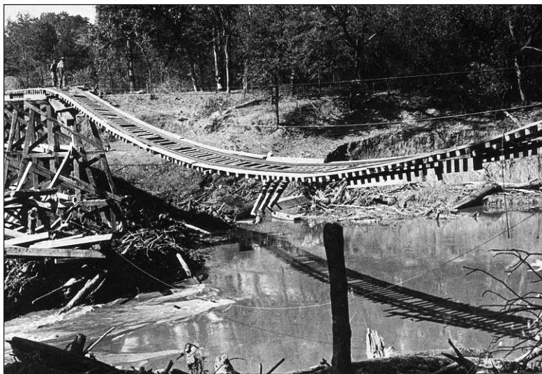
AND THE RAINS CAME: Spring rains stopped work on the Spavinaw waterline at least twice, setting back progress and raising costs.
